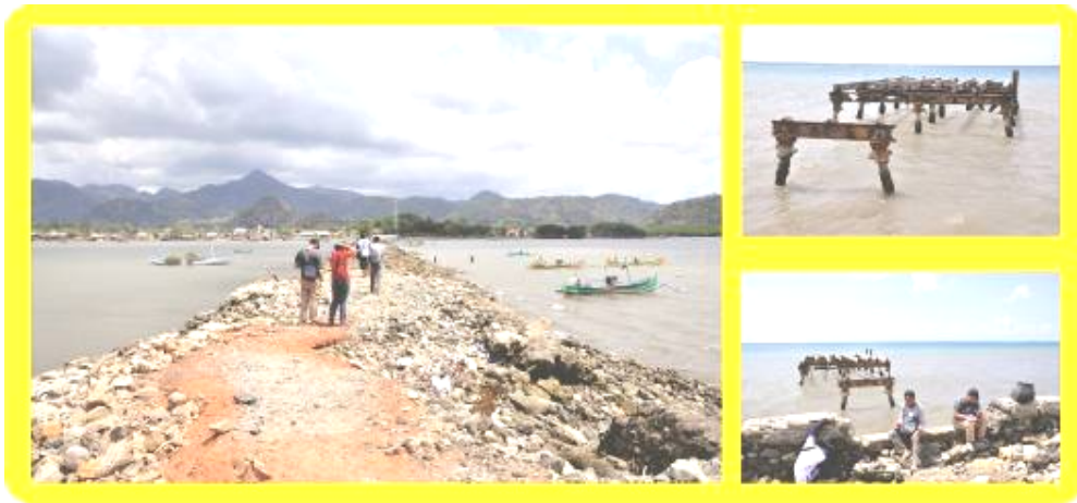
Figure 6. Condition of the colonial-era port in Bawean (Source: Author, 2017)
